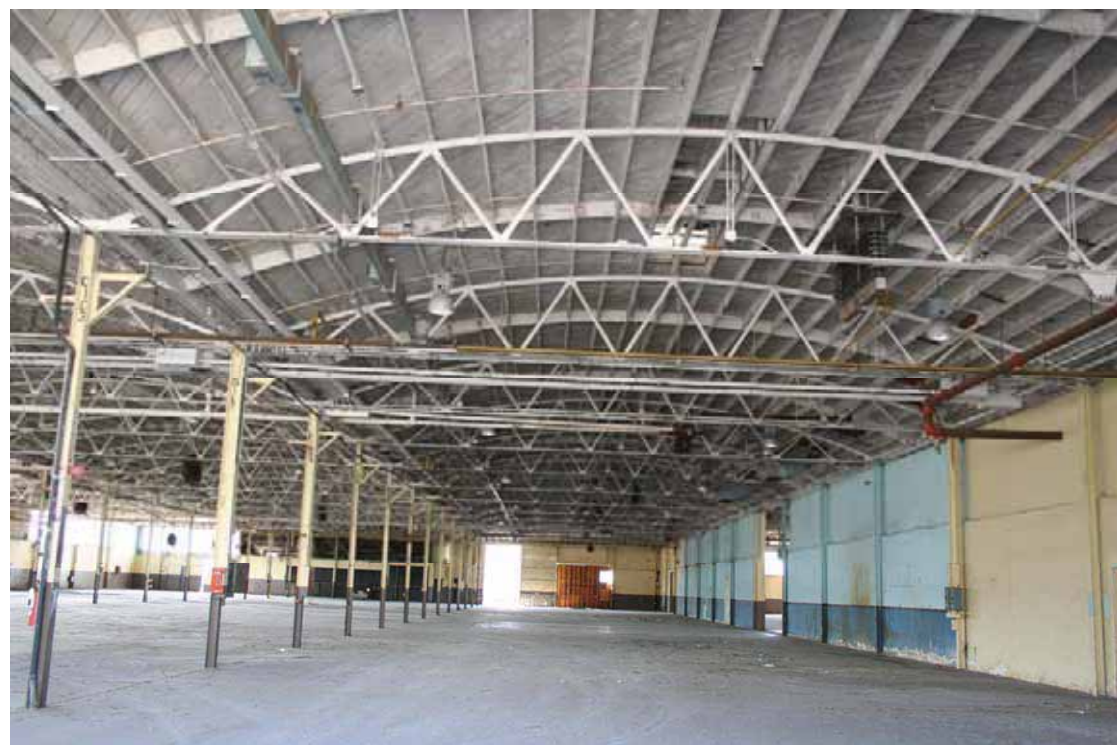
Building 156 – Warehouse, Interior, facing West, the wall on the north (right) is the previously exterior wall of neighboring Building 152, San Diego, California, October 2009.
