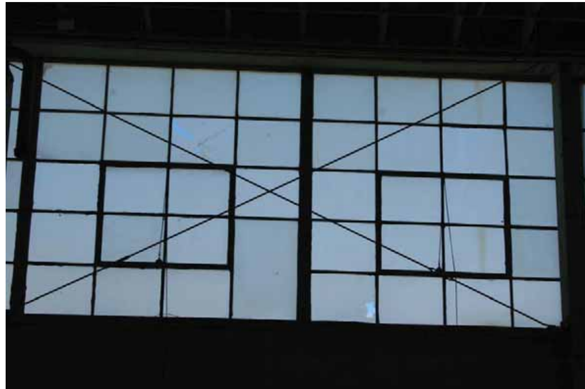
Building 156 – Warehouse Interior, window detail on west elevation, San Diego, California, October 2009.
