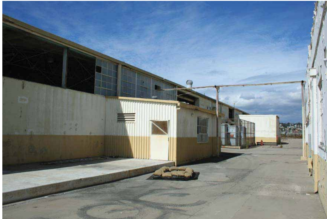
Building 156 – Warehouse, East Elevation, facing Northwest, addition is identified as Building 245, San Diego, California, October 2009.
