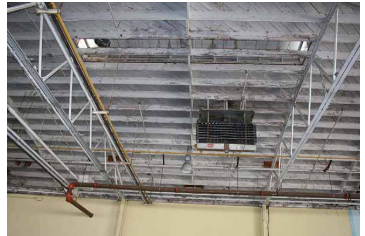
Building 156 – Warehouse Interior, ceiling detail including the roof monitor, San Diego, California, October 2009.
