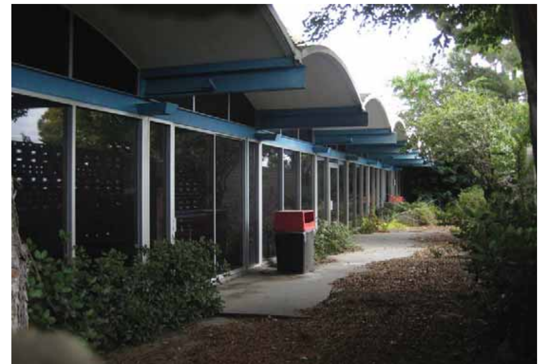
Building 102 - Contracts and Pricing Office, barrel roof over dining area detail, facing Northeast, San Diego, California, October 2009.
