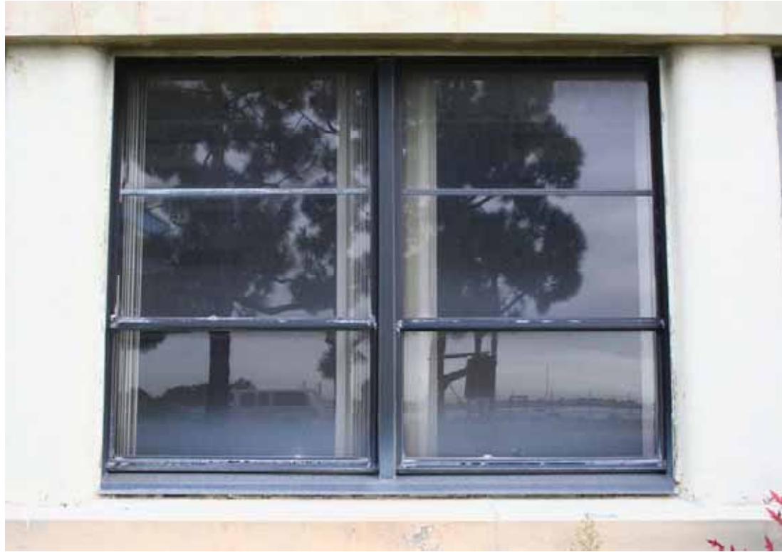
Building 102 - Contracts and Pricing Office, window detail, San Diego, California, October 2009.
