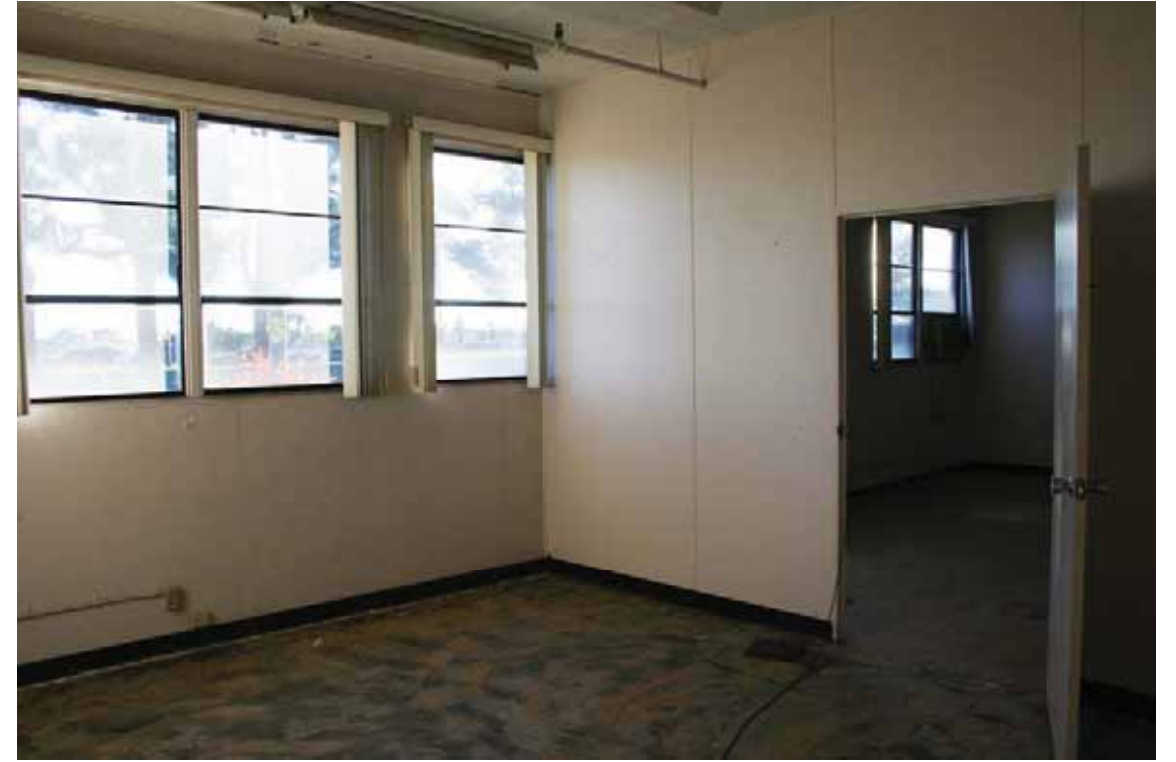
Building 102 - Contracts and Pricing Office Interior, office form detail, facing Southwest, San Diego, California, October 2009.
