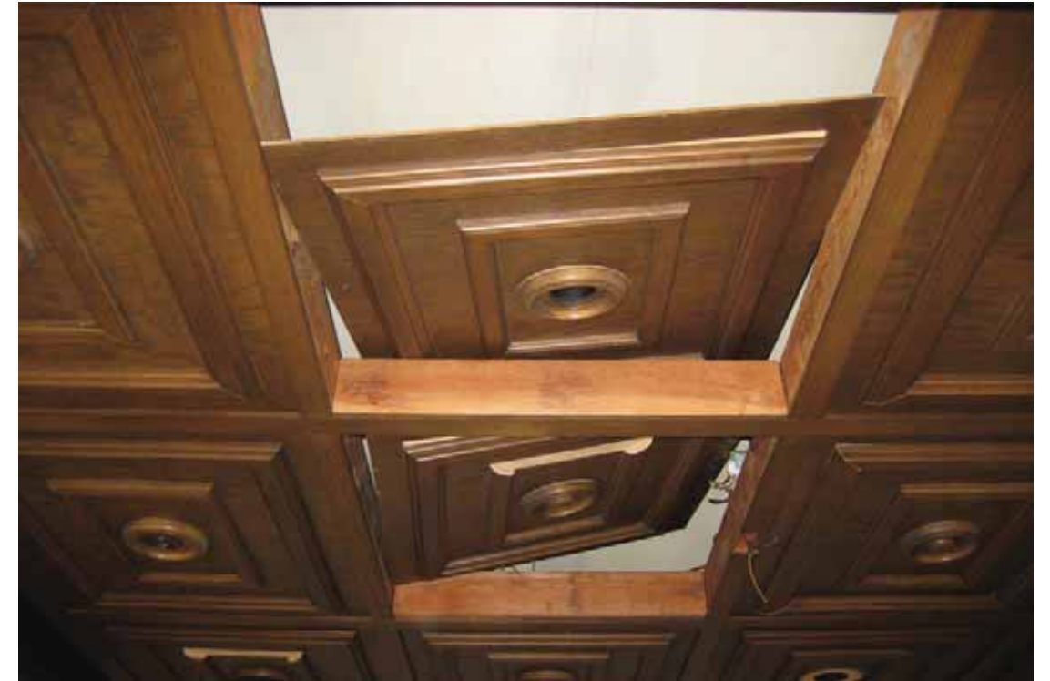
Building 102 - Contracts and Pricing Office Interior, panel ceiling detail, San Diego, California, October 2009.
